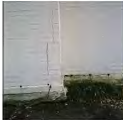
Fig. 8 Cracked foundation on home due to the shrinking and swelling of Houston Black clay it was built upon. Credit: Clay Robinson
